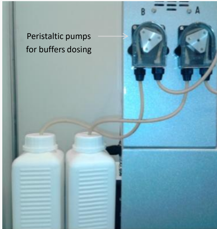
pH control system
