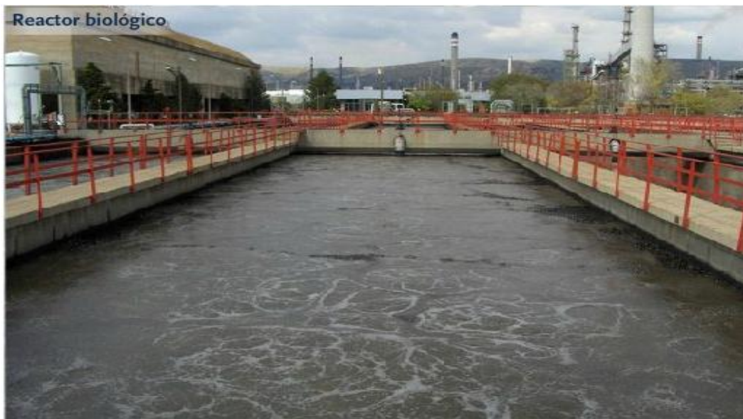
One of the lanes of the biological reactor
